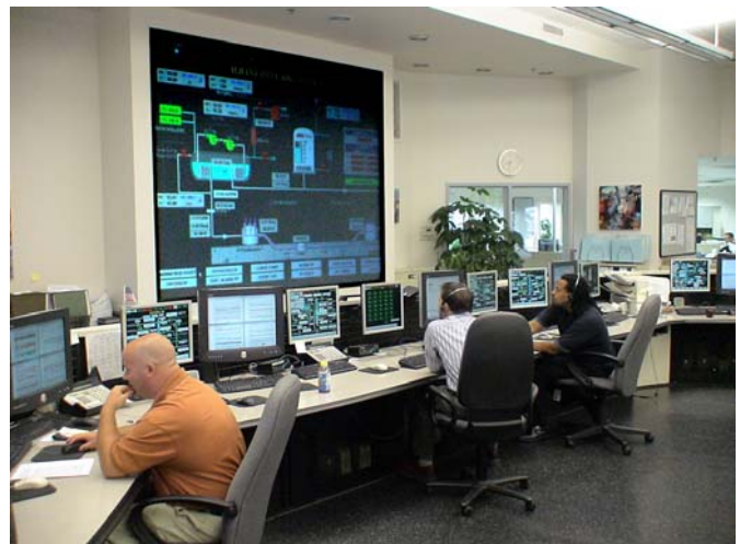
Fig. 3. Remote Operations Center. Albany HTS cable system is monitored from the BOC facility in Bethlehem, PA.
