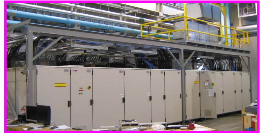
5 MW Converter "Amplifier"
