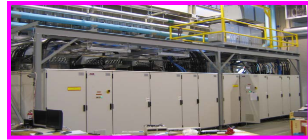
5 MW Converter "Amplifier"
